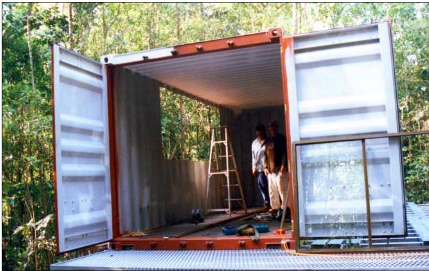
A small angle grinder was all that was needed to cut holes into the sides of the containers. The windows were from an old church.
